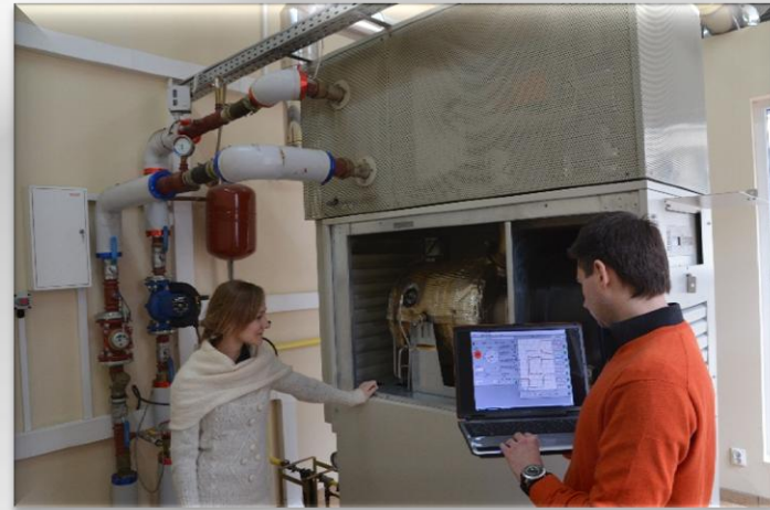
Mikroturbina gazowa Capstone C30
